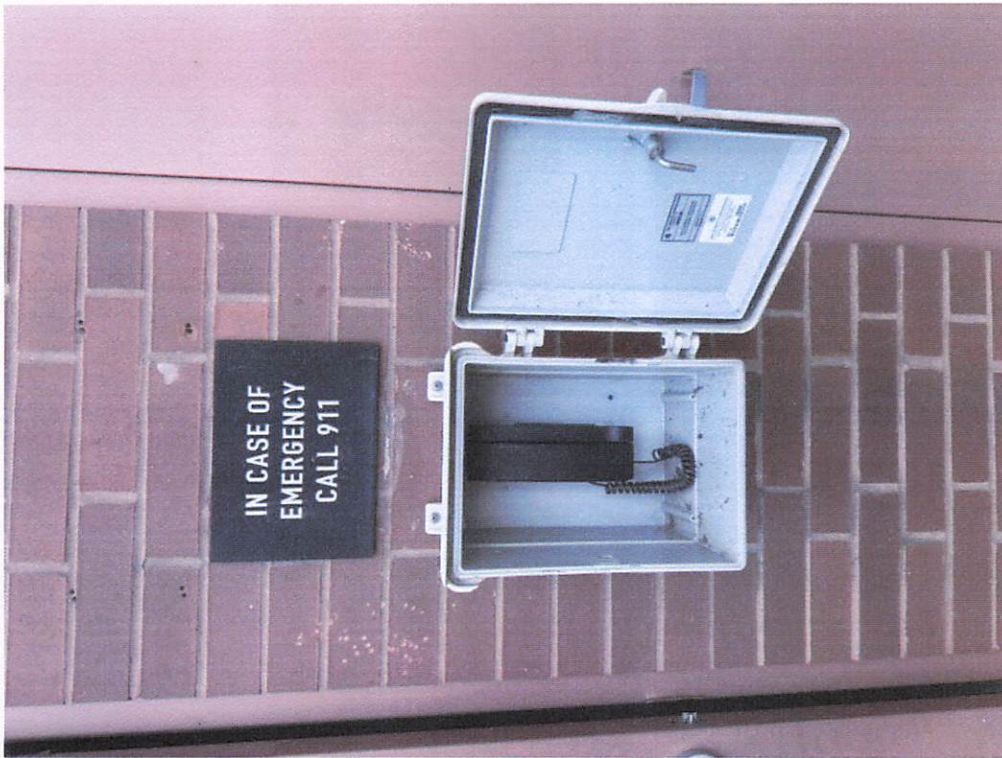
Address for pool at emergency sign missing
