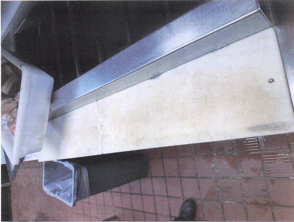
Example violation for inspection report
